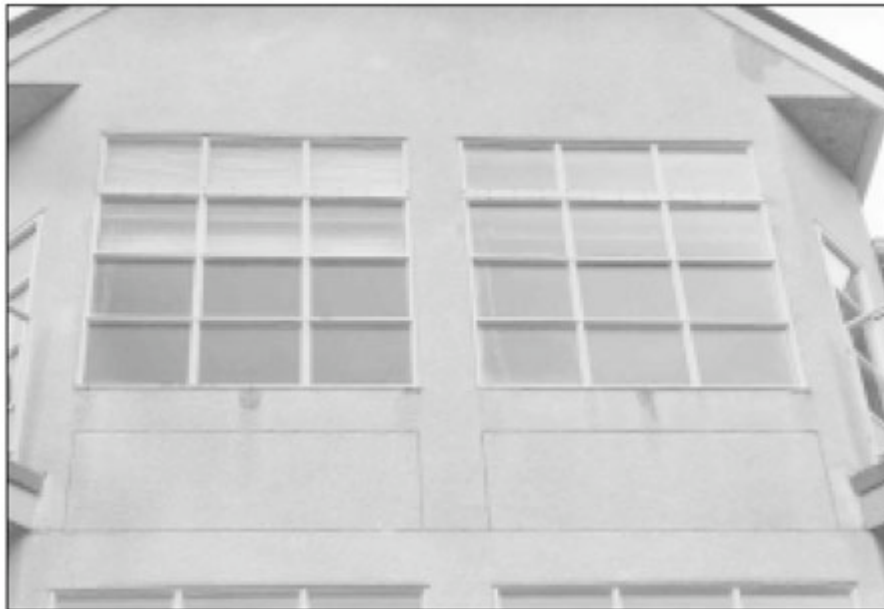
Figure 2. Example of localized wetting as a consequence of ineffective window-seal detail
